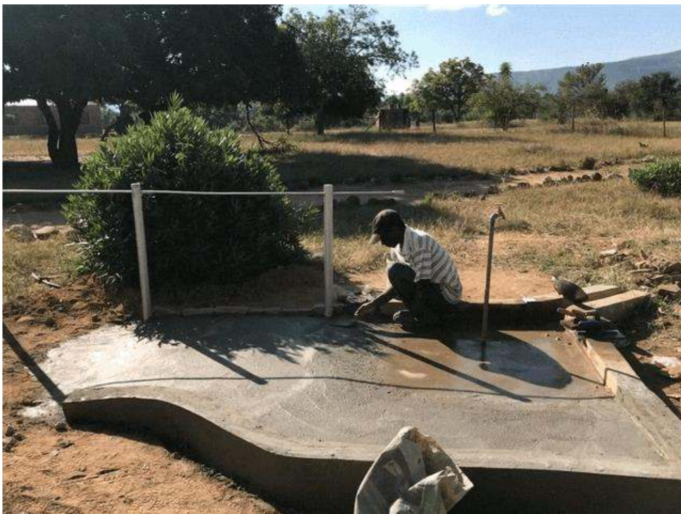
Fig 6 Show construction of a Disability Friendly Stand Pipe for the blind and wheelchair bound
