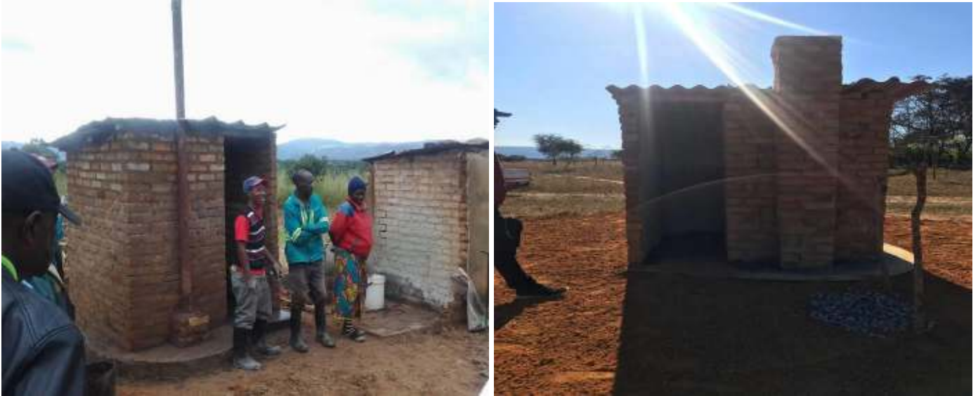
Fig 13 and 14 Construction of Self Sponsored and Grave Yard latrine by an ODF village
